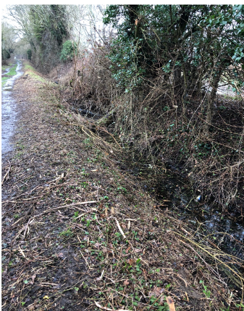
Figure 4.5: Example of the condition of the ditches running parallel to Yarnton/Green Lane
